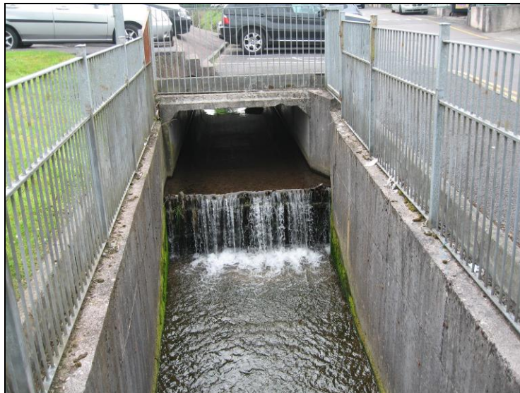
Plate 2: Grange Stream eastern stepped section emerging from culvert in Donnybrook Commercial Park, looking west
