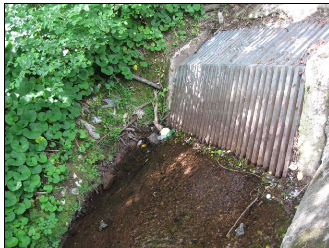
Plate 14: Existing trash screen Tramore River, Lehenaghmore Industrial Estate, looking east
