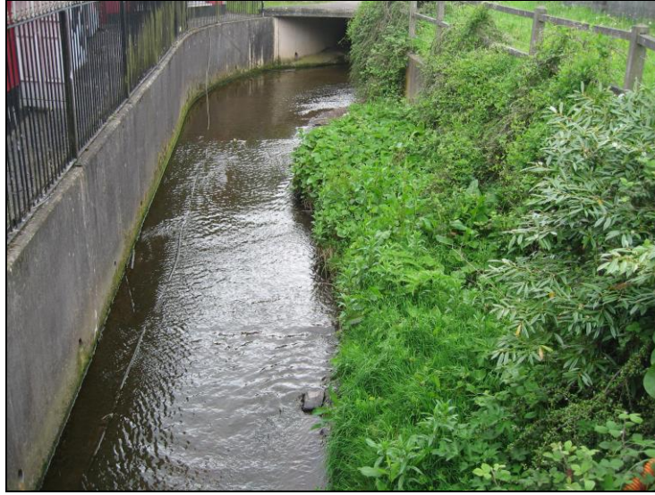
Plate 18: Tramore River emerging from culvert under Togher Road behind Greenwood Estate, looking west
